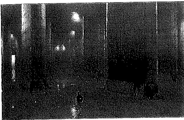
Figure 9. Gigantic pressure-adjusting water tank.
